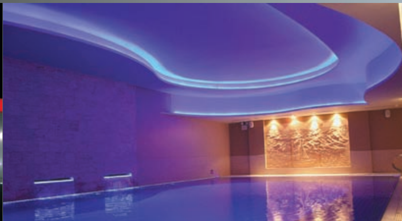
FLPodLED within a cove-lighting and recessed into pool wall - Royal Marine Hotel, Dublin
