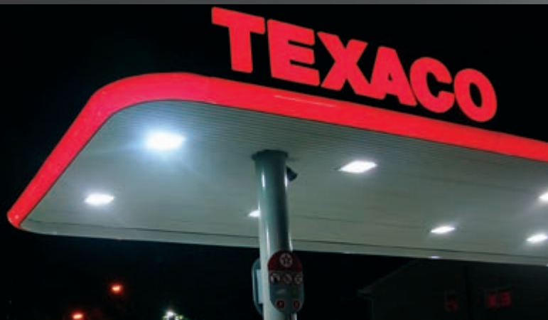
FLPodLED LUX within signage lettering and canopy strip 90% Cost Saving - Texaco Stations Countrywide
