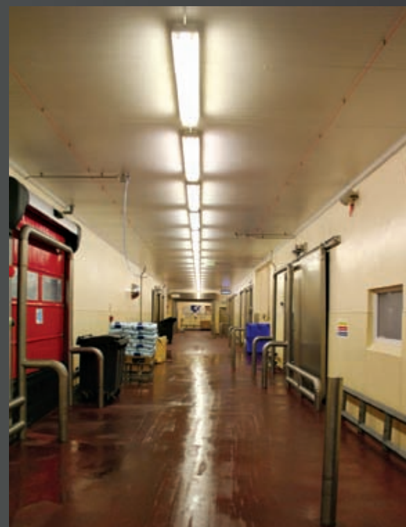
FibreLED Tubes installed within an industrial production facility, running 20hrs/day at a ceiling height of 4metres
